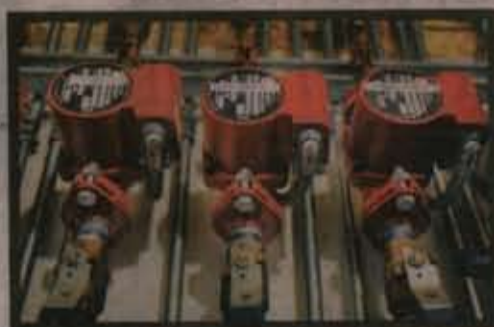
Each room in the house has an individual pump and thermostat for the radiant heating.
